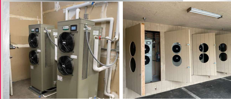
Large Supermarket. Replaced 199,000 Btu/hr natural gas tank water heater with (2) CHP-120 HPWH
