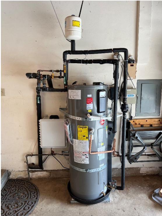
FIGURE 36. PHOTO SHOWING INSTALLED HPWH WITH MONITORING BOX
