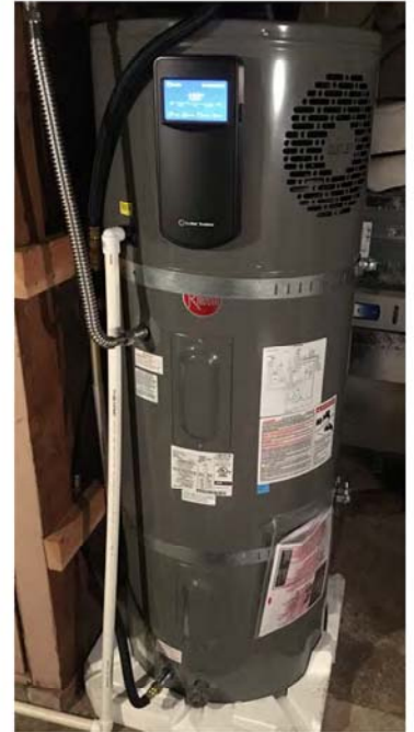
Recent HPWH DIY Install in the basement of Alexi Miller's mother-in-law (Eugene, Oregon)
