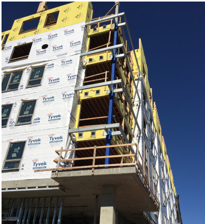
Figure 1: Interior concrete slabs extending unbroken through the thermal envelope and thermally un-broken structural connections turn this multifamily development’s balconies into significant thermal bridges
