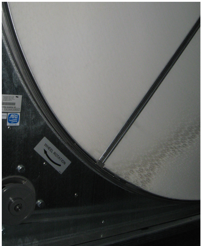
Figure 1: An enthalpy wheel in a central ERV at the Brooks School, North Andover, MA. (Photo credit: Architerra)
